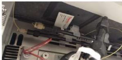
Tag placed flat against the compartment ceiling
