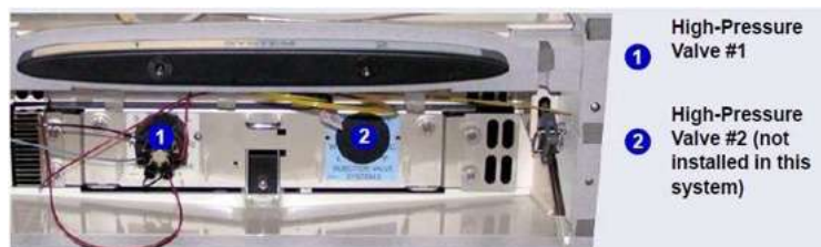
รูปที่ 9-5 High-Pressure Valves #1 and #2 (In DC Lower Compartment)
